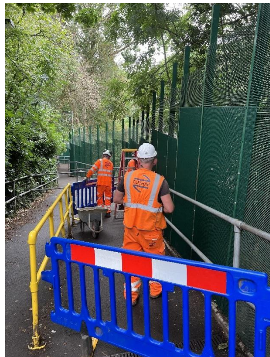
Figure 7 - Use of chapter 8 barriers along public pathway during installation of double skin panels along the 'Blue' section.
