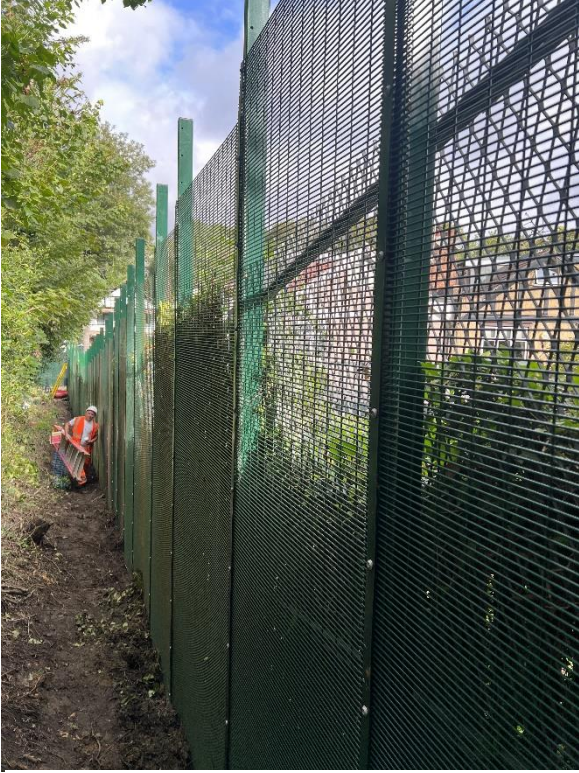
Figure 23 - Installation of single skin 3m fencing along boundary with No.87 Priory Gardens. Existing fencing left in-situ due to resident's outbuildings being fixed to said fence. Furthermore, it was a requirement of the resident to ensure that no vegetation was disturbed within their garden.
