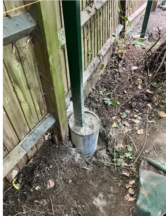
Figure 11 – Using ducts as permanent formwork to enable curation of postcrete footings in difficult ground conditions.
