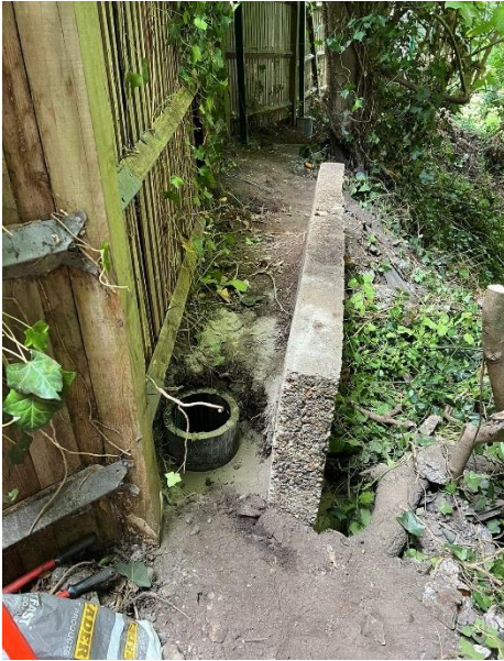
Figure 13 - Example of the difficult digging conditions with minimal space to use hand tools effectively.
