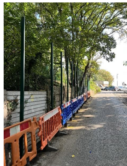
Figure 32 - Chapter 8 barriers sectioning off newly installed posts at the end of the shift.
