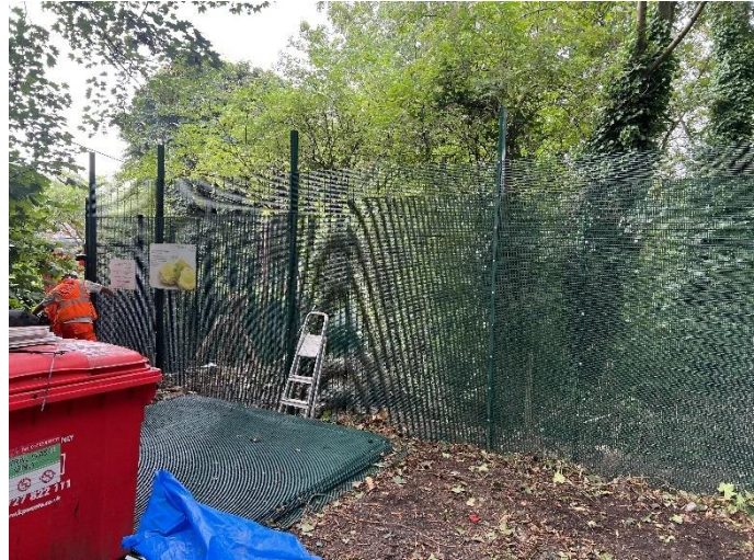
Figure 14 - New double skin prison mesh fencing installed and existing pub car park signage fixed back to new fence.
