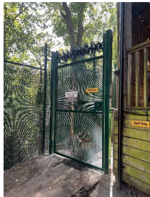
Figure 16 - New standard single gate topped with anti-climb raptors installed to pub staff entrance to enhance security.
