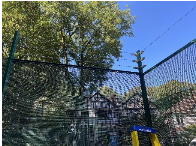
Figure 28 - Installation of 3-strand barbed wire to the rear of cafe Noir coffee shop at the priory gardens entrance to Highgate station.
