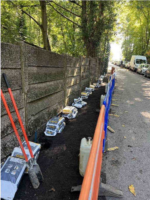
Figure 33 - Excavations along car park boundary, postcrete loaded out, also showing existing concrete fencing to be removed.
