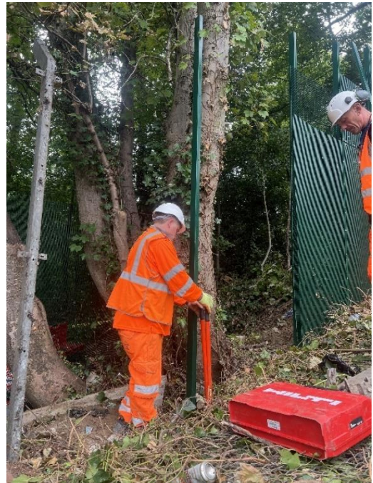
Figure 30 - Installation of final panels along the yellow run, severe sloping ground levels next to the entrance of the station car park.
